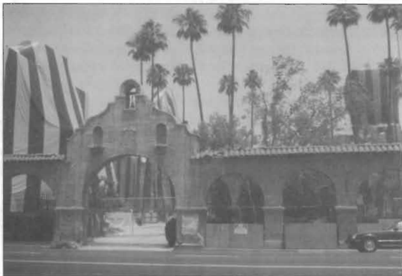
The Mission Inn from Seventh Street during restoration, c. 1988 (Courtesy of the Riverside Public Library)
